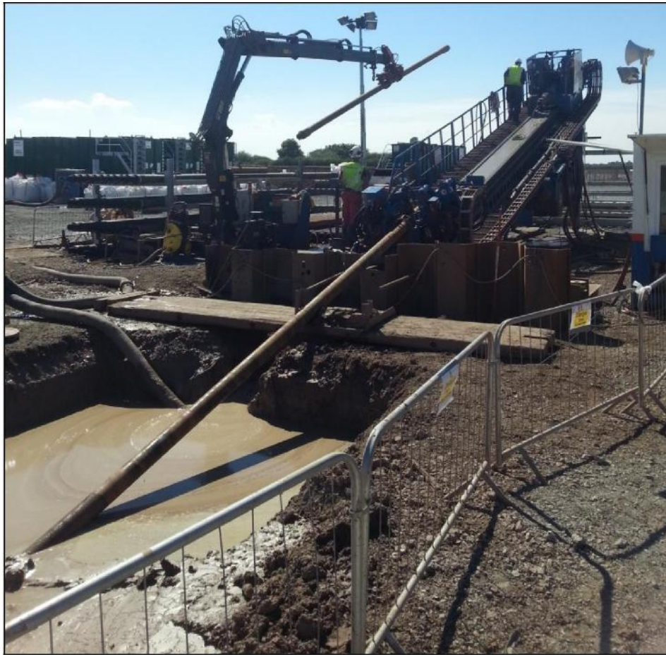
Figure 4.18: HDD rig carrying out landfall works at the Westermost Rough offshore wind farm
